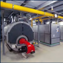
Energy efficient combined heat and power plants (CHP) in our plant in Teisnach, GER
