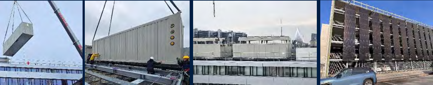
Usage of waste heat - Heat pumps for R&S data center (4 x 300 kW) in R&S Headquarters
